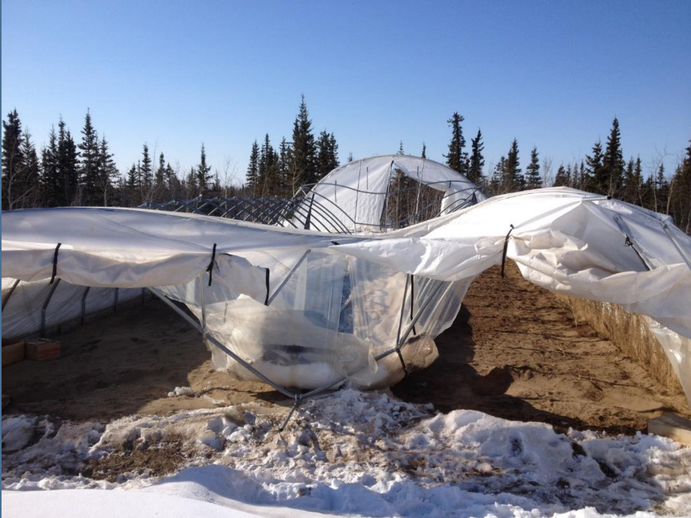
An early and heavy wet snow collapsed this high tunnel.
